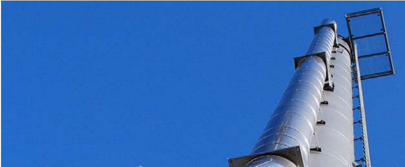
Air purification exhaust gas treatment & etc.
